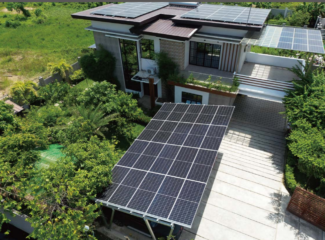
Metal Roof & Carport Mount-Philippines
